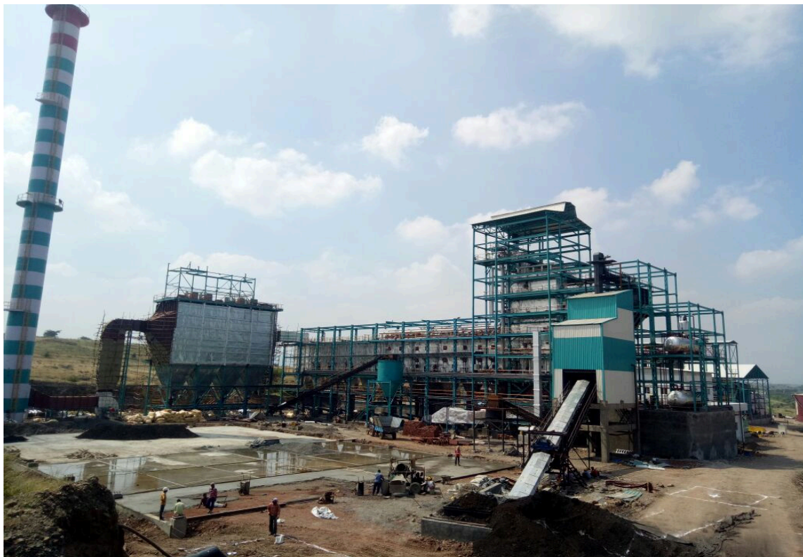
Sharayu Agro Industries Limited (Spent Wash Incineration Boiler)
